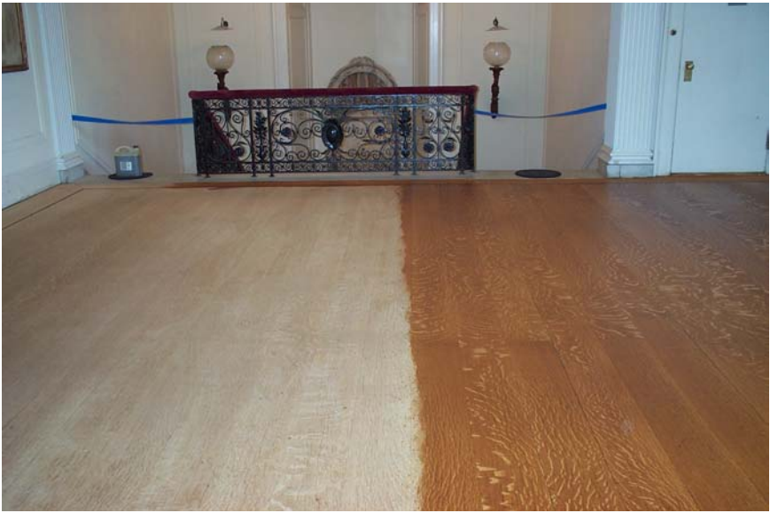
In this series of photos we see the progression of the finish as it is applied to the foyer floors. Please note the uniformity of color and the lack of distortion that was in the original finish prior to its removal.
